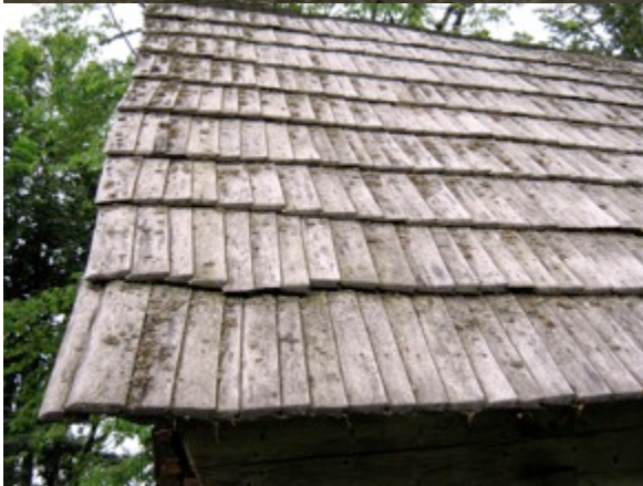
Top: new roof of thin shingles on the museum Below: Traian's traditional shingles on his storehouse
